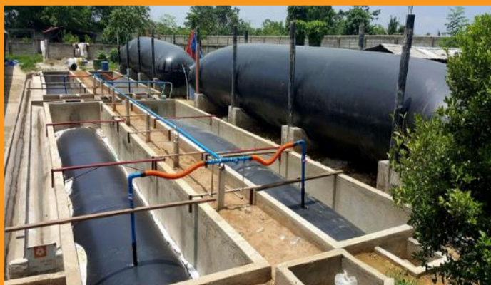
AD System Installed at Bulucan Farm Cooperative
