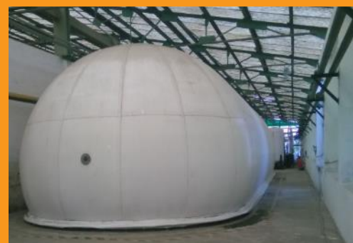
Flexible storage unit for upgraded biogas
