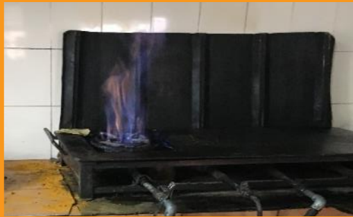
One of the kitchen's biogas powered stoves
